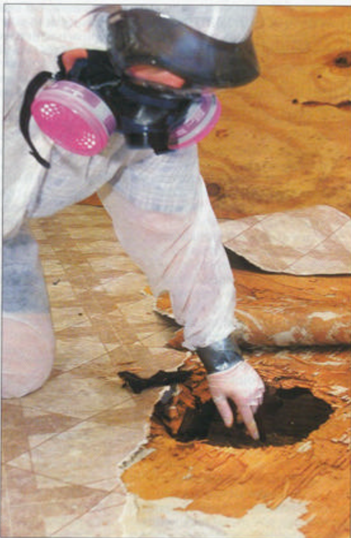
A contractor garbed in an environmental protection suit inspects mold damage to a house in Flour Bluff, Texas.
